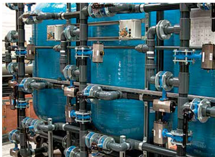
Picture supplied courtesy of Sterling Hydrotec.
